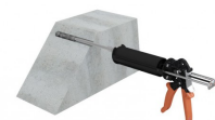
Fill the hole to half or two thirds. Withdrawing the nozzles with each pump.
